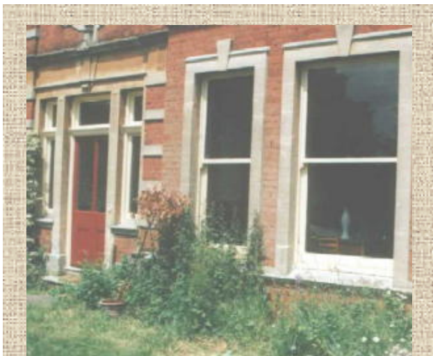
eco-paints on doors and sash windows: Redfield has changed from waterproof paint to eco-paints on all 200 windows on the house and stable block; only natural, breathable materials are now used – for example lime mortars and linseed oil putty instead of cement mortars or mastics.
